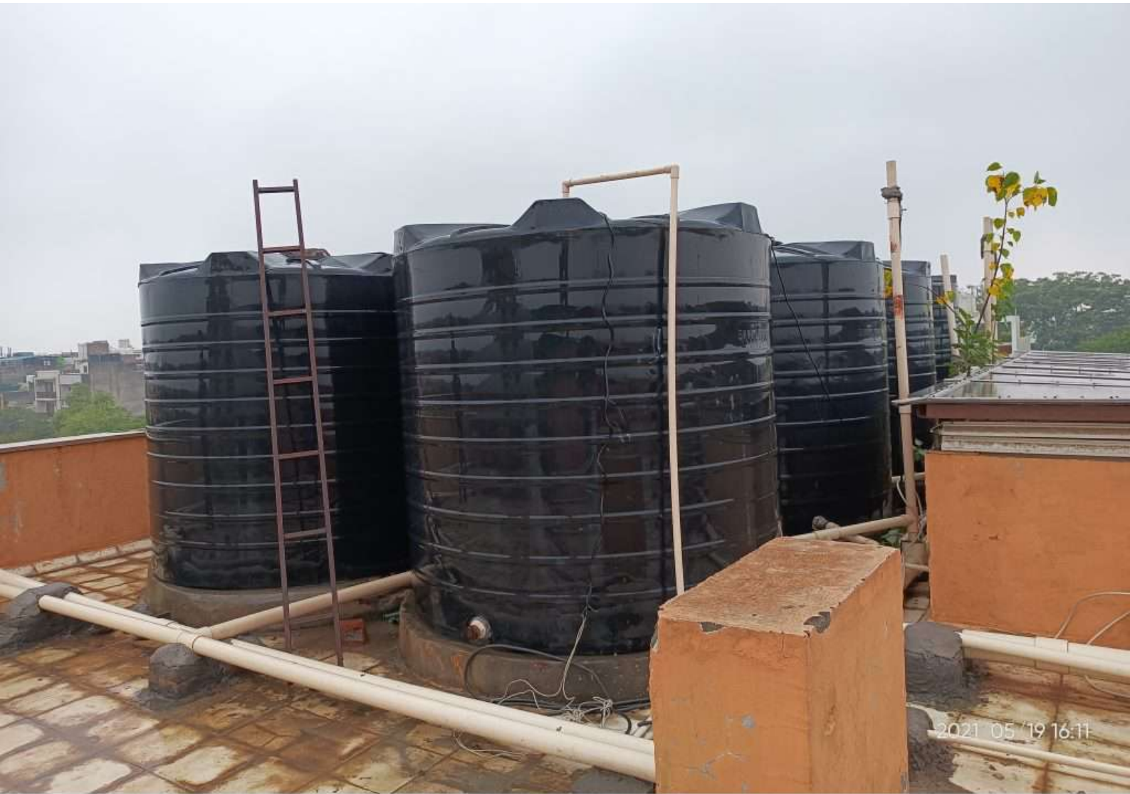
Water Tanks, Ramanujan College
