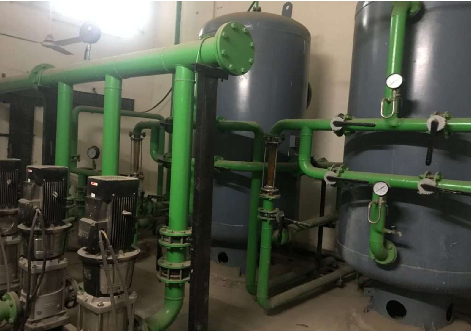
Water Treatment Plant, Ramanujan College
